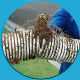
Existing Drainage System Failure?
